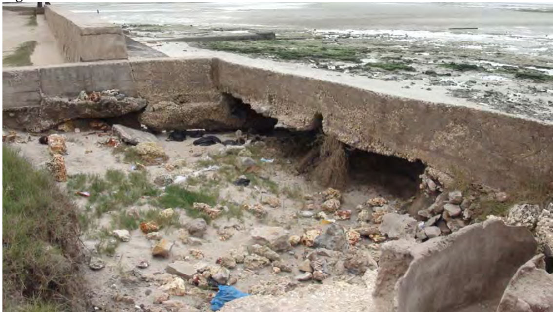
Figure 7: Evidence of severe degradation in sea wall along Ocean road.
