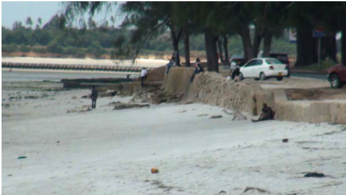
Figures 4-5: Evidence of water movement towards the wall and wall degradation along ocean road.
