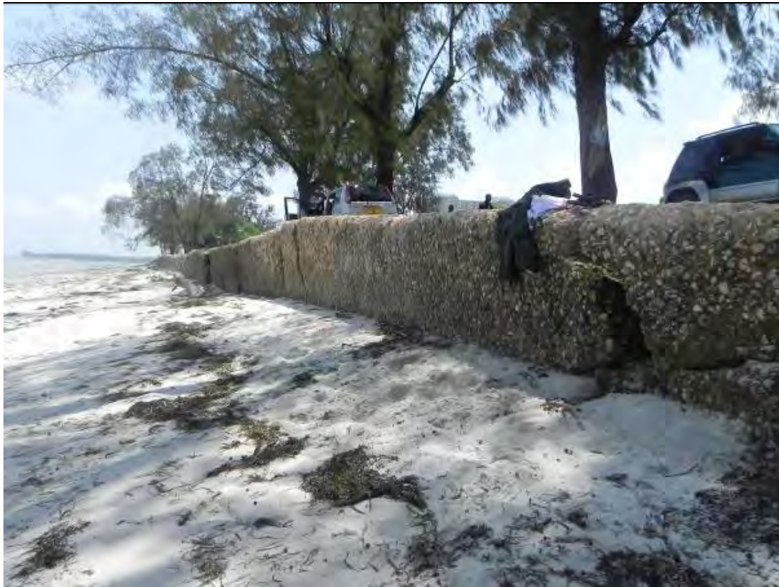
Figure 2-3: Current Situation Of The Sea Wall In Dar Es Salaam To Be Re-Constructed
