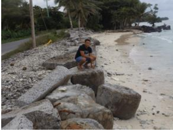
figure 9 pal section of malem road. mass concrete bags, loose boulders and broken concrete, placed randomly to reduce surge impact and prevent wave overtopping and erosion of road (source of photo: simpson abraham, july 2015)
