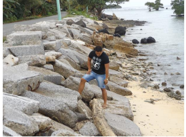
figure 10 mosral section of malem road. existing dumped concrete rubble here will need to be removed. a proper double layer rock armour (revetment) is required to protect the critically exposed road. a low reef flat breakwater to 'stabilize' shoreline will also be required further south to prevent outflanking and downdrift erosion. ((ksmp, 2014; source of photo: simpson, july 2015)
