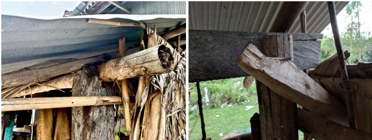
Figure 18 “Example of poor joint construction with inadequate materials and construction quality. Example of poor joint construction.”
