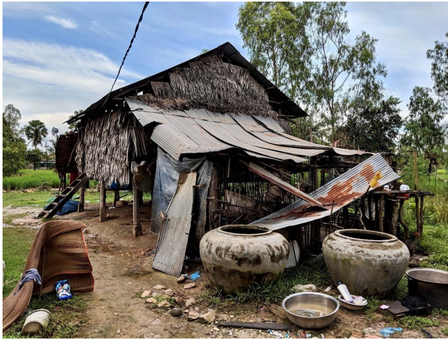
Figure 4 “Typical example of poorly constructed traditional house. This house is located in the Prey Thom commune.”
