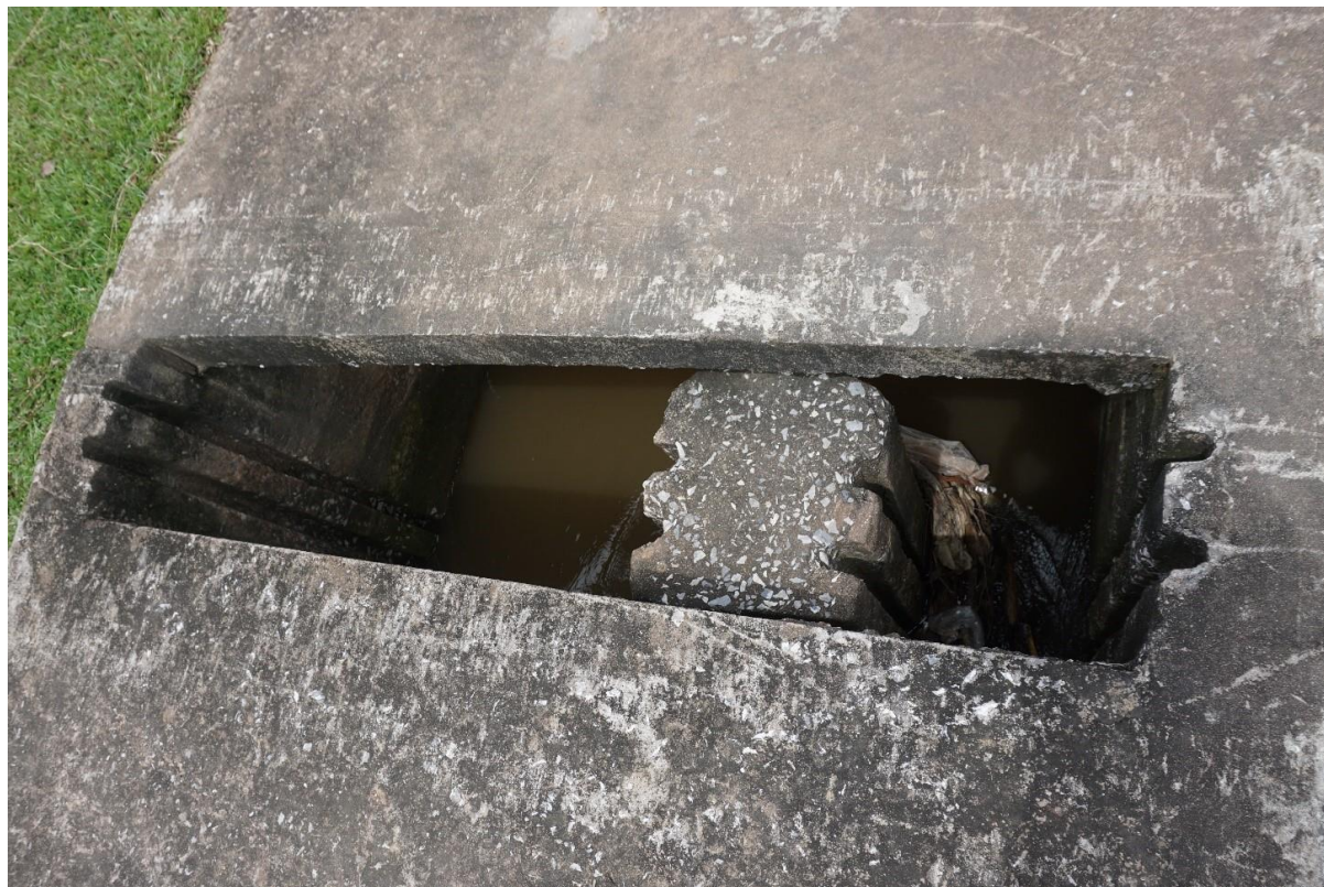
Figure 4 “Missing spindle in gate 1”
