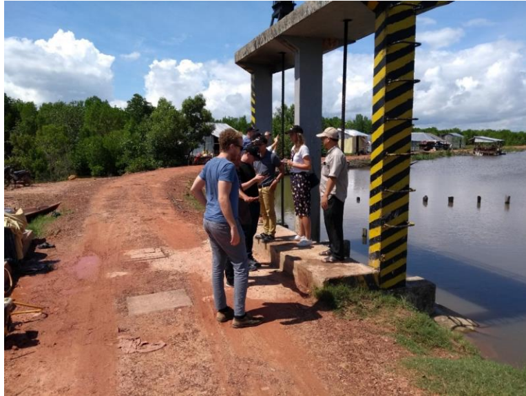
Figure 3 “Photo 2 – note the steel rungs projecting from the near upright of the sluice gate structure. Some of these were observed to have rusted through. A new steel ladder should be provided fixed securely into the concrete uprights using brackets.”
