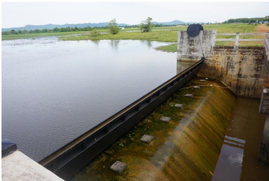
Figure 7 “O Thmar reservoir automatic radial gate and spillway”
