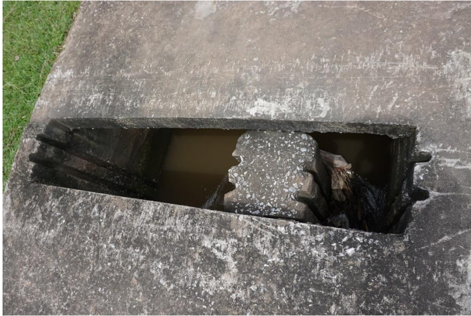
Figure 16 “Missing gate = water gate 1”
