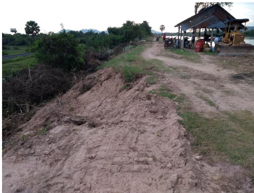
Figure 3 “View along the crest of the dam showing eroded embankment face and vegetation on the downside of the dam”
