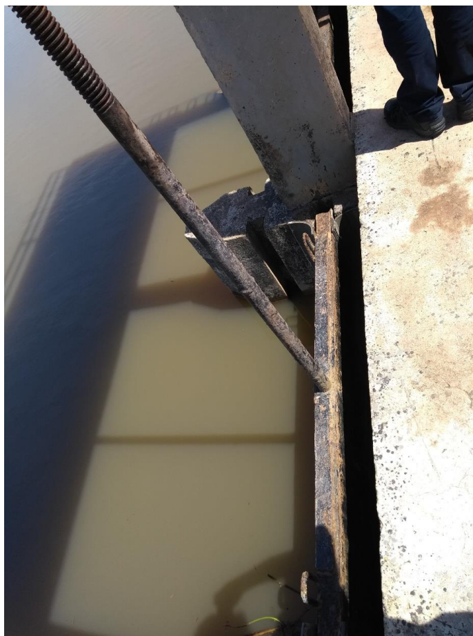
Figure 2 “Photo 1 – Existing sluice gate. Note the stop board slots on the outside of the structure (arrowed). When boards are placed in these down to the cill this will enable the gates to be removed and refurbished while water is prevented from passing through the structure”
