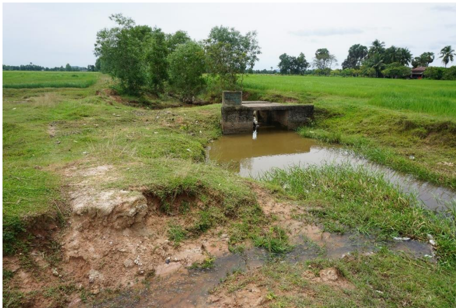
Figure 15 “Erosion embankments water gate 1”
