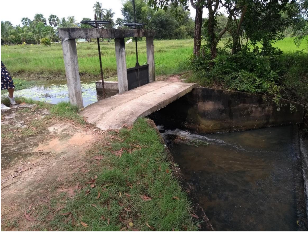
Figure 2 “Watergate 2 eroding embankment upstream and downstream embankment in Angkaol Commune”
