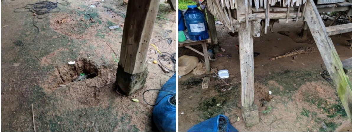
Figure 16 “Closeup of foundation failure identified in Figure 10. Foundation not secured into ground with evidence of previous failure.”
