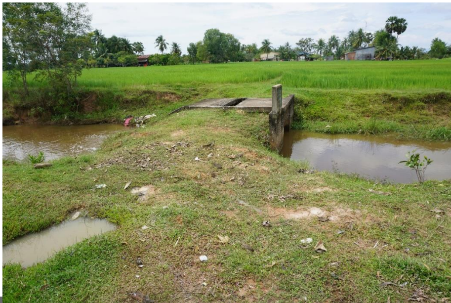
Figure 17 “Eroded embankments around water gate 1”
