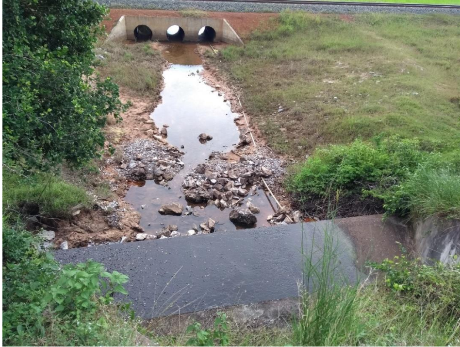
Figure 7 “View downstream from the main outlet sluice showing the apron and the railway culverts.”
