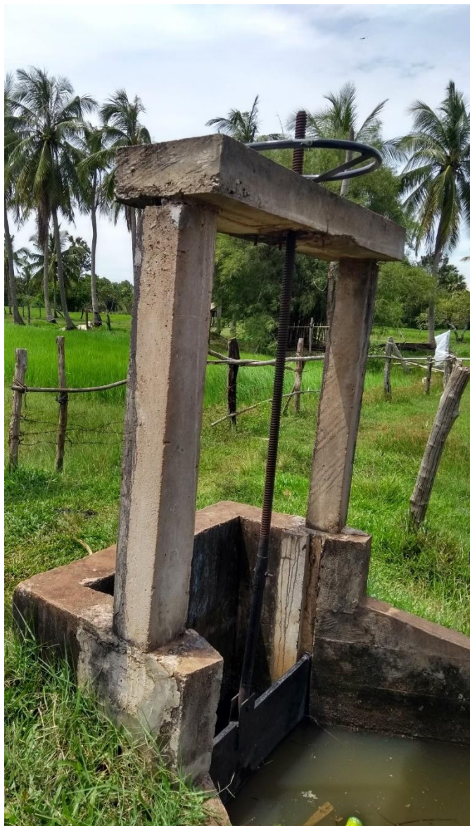
Figure 3 “Watergate 3 scour underneath the water gate in Angkaol Commune”
