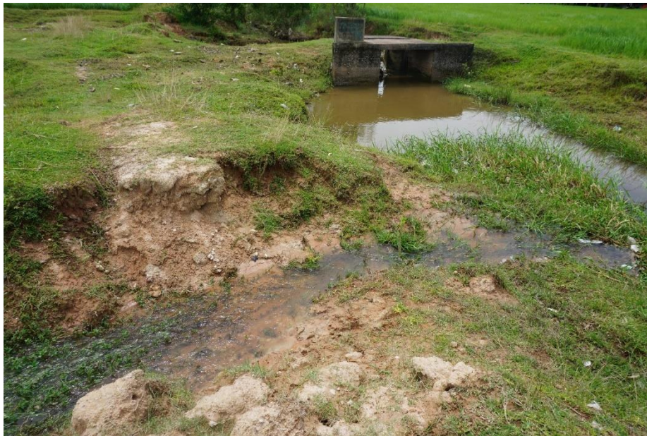
Figure 14 “Erosion upstream water gate 1”
