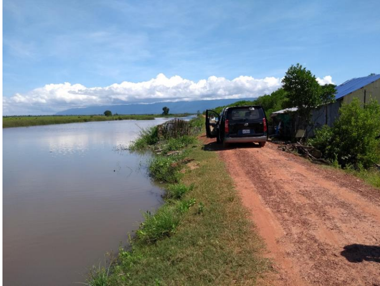
Figure 4 “Photo 3 – The existing shallow embankment showing the limited width for vehicle access and the drainage canal to the left (landward) side. Informal settlement building on the right-hand side.”
