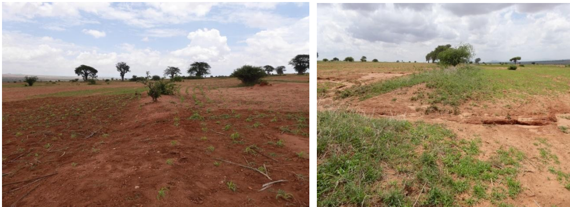
Figure 6: A bund being farmed (left side) and Spot failure along a bund Right side) (Source: Field survey during the preliminary project design)
