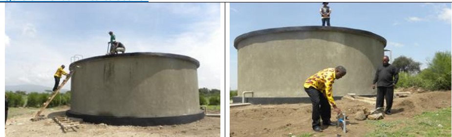
Water storage tank constructed at Meseraniuu Village through a decentralized climate funds.
