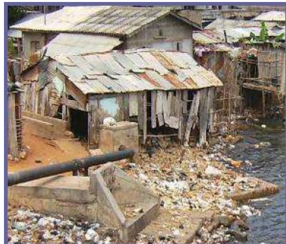
Figure 2.1 : outlet of rain waters or waste waters’ main sewer, drink water conduits stripped by erosion in an unhealthy environment on the banks of Cotonou lagoon
