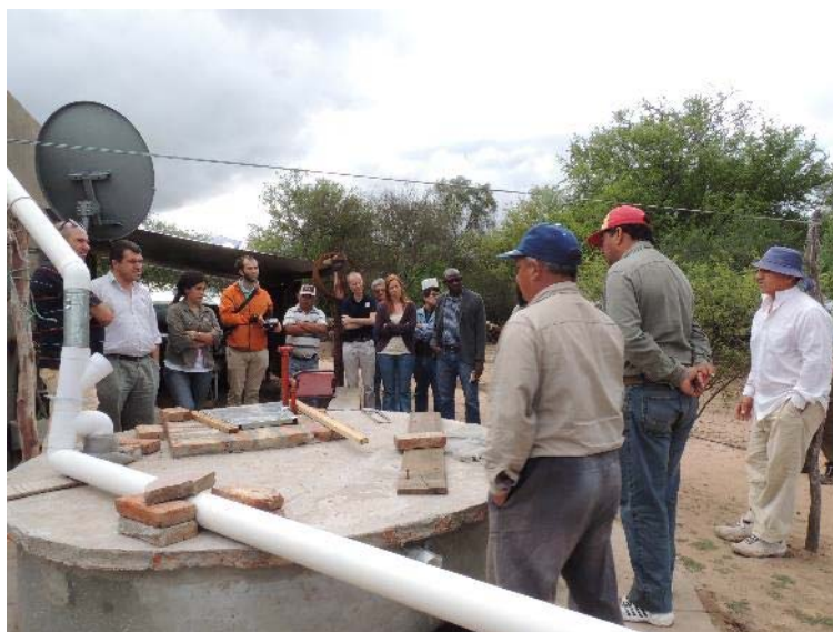
Figure 3 : Example of a household-level water harvesting technology built by beneficiaries in Argentina
