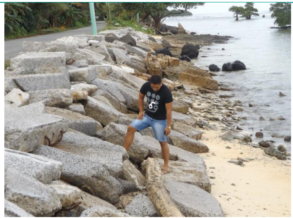
Paal section of the coastal road. Existing dumped concrete rubble. A low reef flat breakwater to 'stabilize' shoreline will also be required further south to prevent outflanking and downdrift erosion. (photo credit: Simpson Abraham, 2015)
