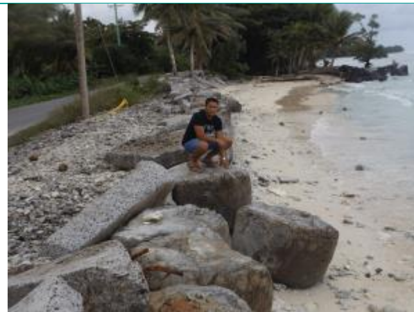
Mosral section of Malem road. mass concrete bags, loose boulders, and broken concrete, placed randomly to reduce surge impact and prevent wave overtopping and erosion of road (photo credit: Simpson Abraham, 2015)
