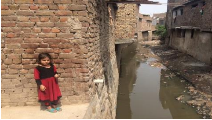
Figure 11: Drainage channels closed-in by houses and filled with waste in target communities in Rawalpindi – flood levels reach four meters above the channel banks, which is the 2 nd floor of houses.
