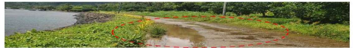
Infrastructure site 4: Salimu/ Musumusu rockwall – rocks are crumbling into wetlands and water is collecting on the road
