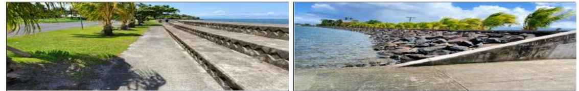
Infrastructure site 3: Vaiala seawall – no visible defects (landside view, left; seaside view, right)
