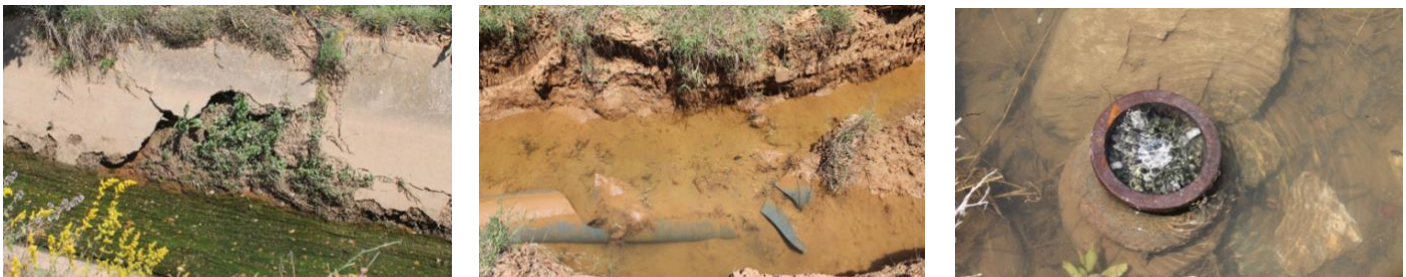
Figure 8: left to right: i) right main channel; ii) burst pipe on the right channel; iii) obsolete flooded hydrant (Source: FAO, 2021)
