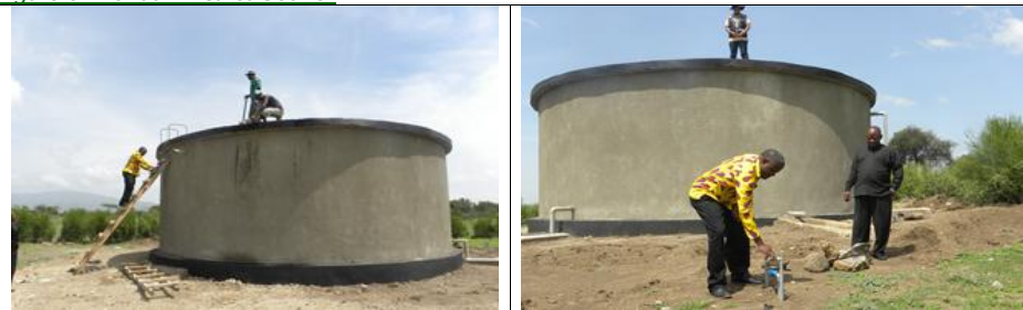
Water storage tank constructed at Meseraniuu Village through a decentralized climate funds.
