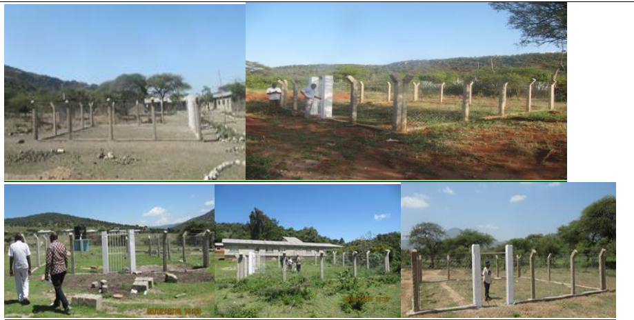
The Installed Meteorological Stations at Ngaresero Primary School, Digodigo Secondary School, district Council Headquarter, Ololosokuan and Malambo.
