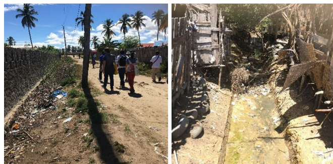
Figure 9: Drainage conditions in Morondava
