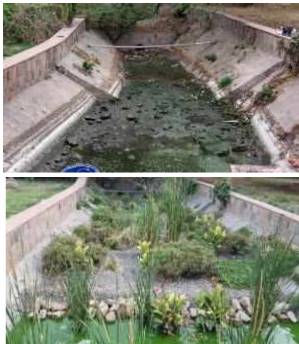
Figure 10 – Outfalls Conversion of a drainage canal into a subsurface flow constructed wetland
