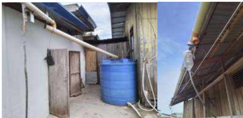
Figure 5. Existing rainwater harvesting systems, Sitangkai
