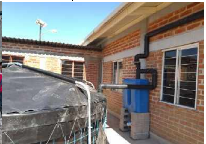
RWH system in the INPI shelter, Las Tapias
