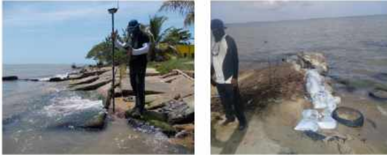
Figure 16: (left) Destruction of the facility by erosion in Dangriga. (right) Type of ineffective defense structure
