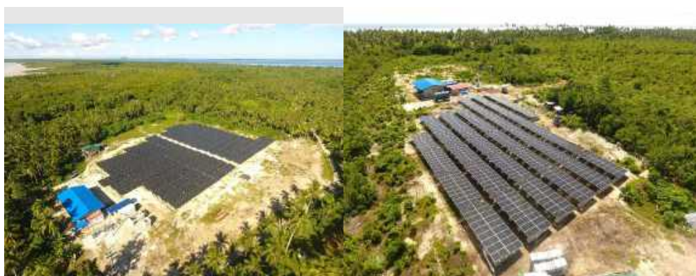
Figure 22. Photovoltaic plants and diesel generators deployed by the RETS project in Sibutu and Sitangkai, as of October 2021. Source: The RETS project
