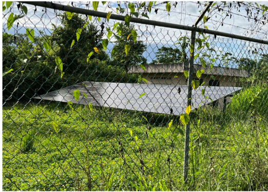
Figure 23: Example of Solar Panels used for Water Pump (Source: Site visit 2023).
