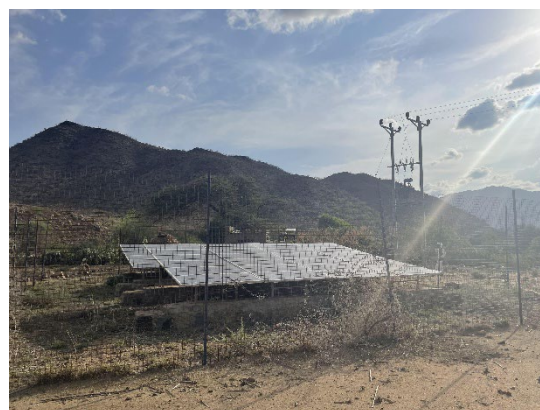
Image 2 Solar power irrigated pumps and reservoir in Fiza, Habero
