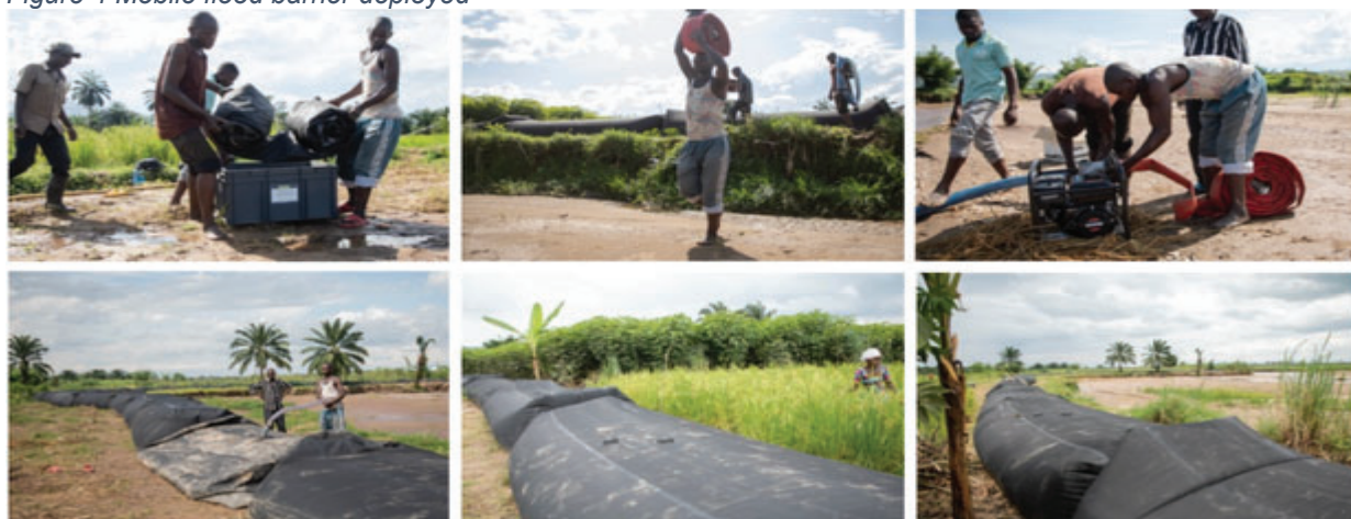
Figure 4 Mobile flood barrier deployed
