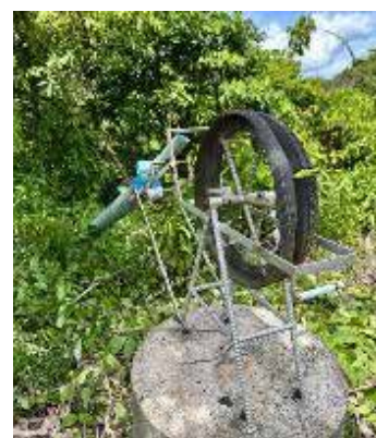
Figure 3. Manual water-pump mechanism installed at the pond site
