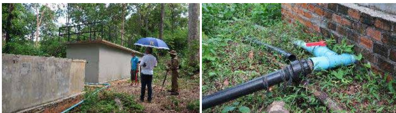
Figure 1. Partially damaged water treatment plant and main water pipe
