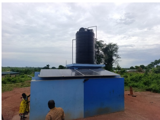
(a) Solar high-voltage system
