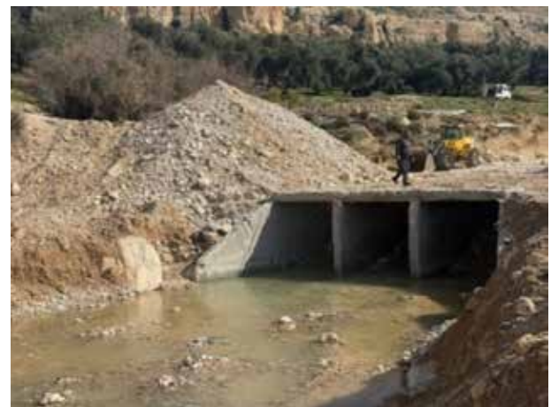
FIGURE 42: INFRASTRUCTURE DISRUPTION IN WADI AL-KARAK
