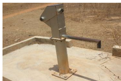
Image 10. Broken Borehole Handle in Zaazi, Northern Region
