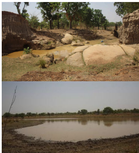
Image 11. Broken dam embankment and diminishing dam water in Goli, Upper West Region
